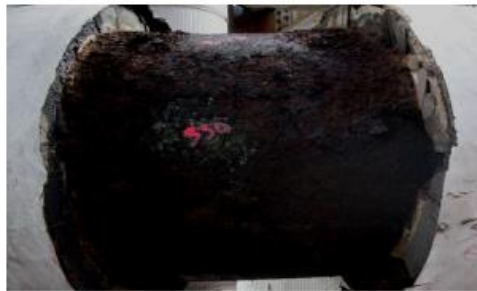
Figure 12: CUI becomes a significant issue when insulation plugs are removed but not replaced and rescaled again (PetroChem Inspection Services Inc, used with permission)
