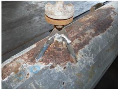
Figure 3: CUI as induced on inorganic zinc coating after working for 8 years in a coastal industrial atmosphere: Note the steam inlet nozzle and the effect of water ingress around it. © National Corrosion Association (NACE) ®
